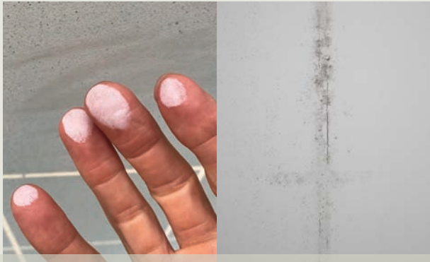
// Chalking and cracking of a backsheet
