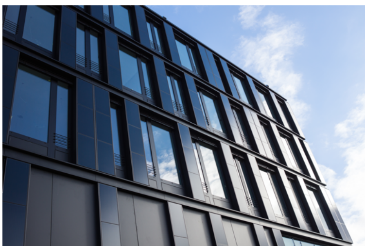
Façade with integrated CIGS thin-film solar modules at the ZSW institute building in Stuttgart, Germany (Photo: ZSW)
