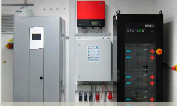
// PV storage system test bed
